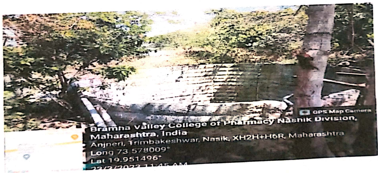
Photograph of Water Well
