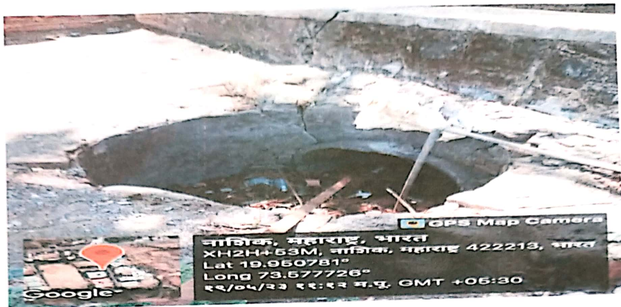
Photograph of Water Drainage system
